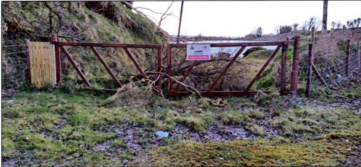
Figure 3: Lack of adequate fencing as required under Condition No. 20 of Reg. Ref. 07/267.
